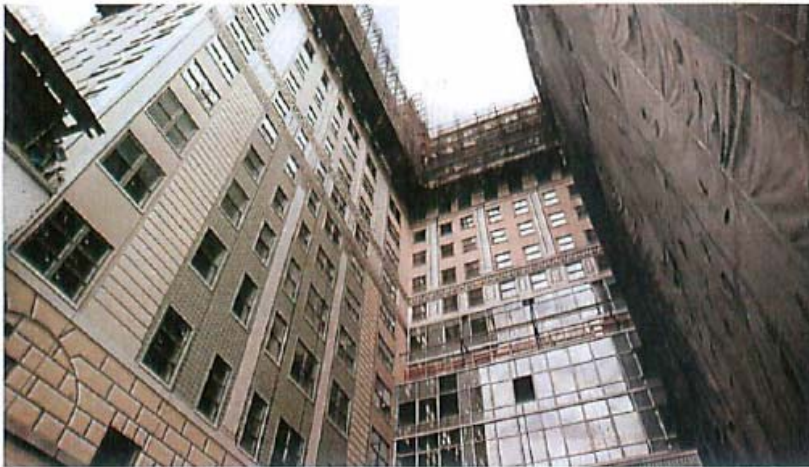
Construction continued on the conversion this year at 110 Livingston in Brooklyn, which will have four new glass-faced floors above the original 1926 structure, seen here from an interior courtyard.
